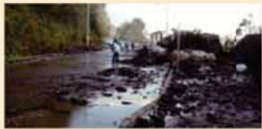
Damage by wave going over an embankment (Route 55)
