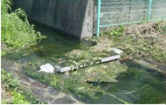
刈草、野菜くず、ビニル袋等によりすぐに目詰まり (Clogging quickly due to cut grass, vegetable scraps, plastic bags, etc.)
