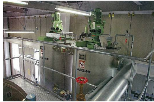
凝集材混和槽
